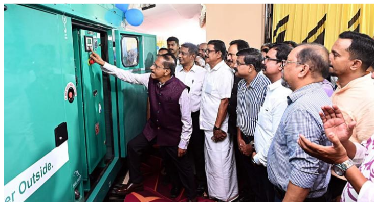
Donated a 250 KVA Diesel Generator to Thanal Dialysis Centre, Vatakara, Kozhikode
