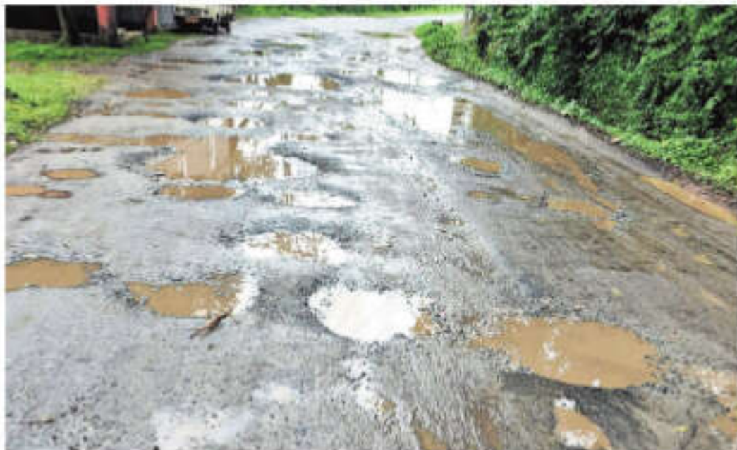
The condition of Virajpet-Madikeri Road | EXPRESS
